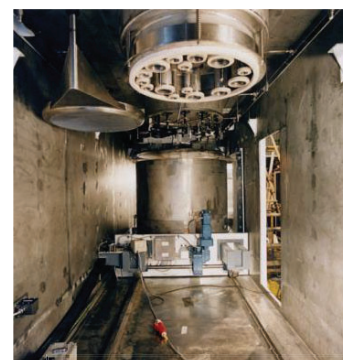
Figure 3: Processing container (Module 2)
