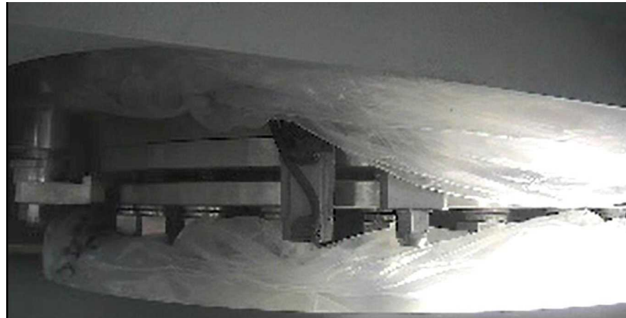
Connection completed between telescopic equipment & connection structure / connection pipe (Scene from above)
